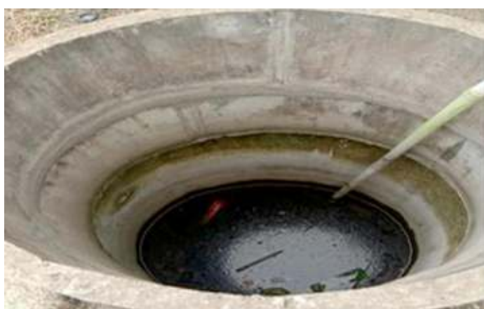
(SP Palu documentation, condition of community water sources polluted by coal waste and dust)
