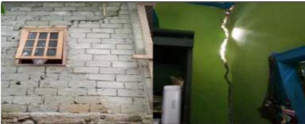
Do SP Sintuwuraya Poso Documentation: Community houses damaged by dredging and bombing activities on the Poso riverbed by the PLTA Poso 1 and 2 in Sulewana village
