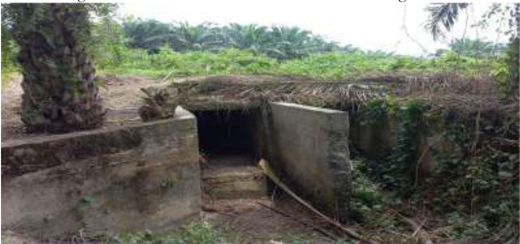
(Solidaritas Perempuan Documentation: Water gates to drain the swamps planned be transmigration locations)
